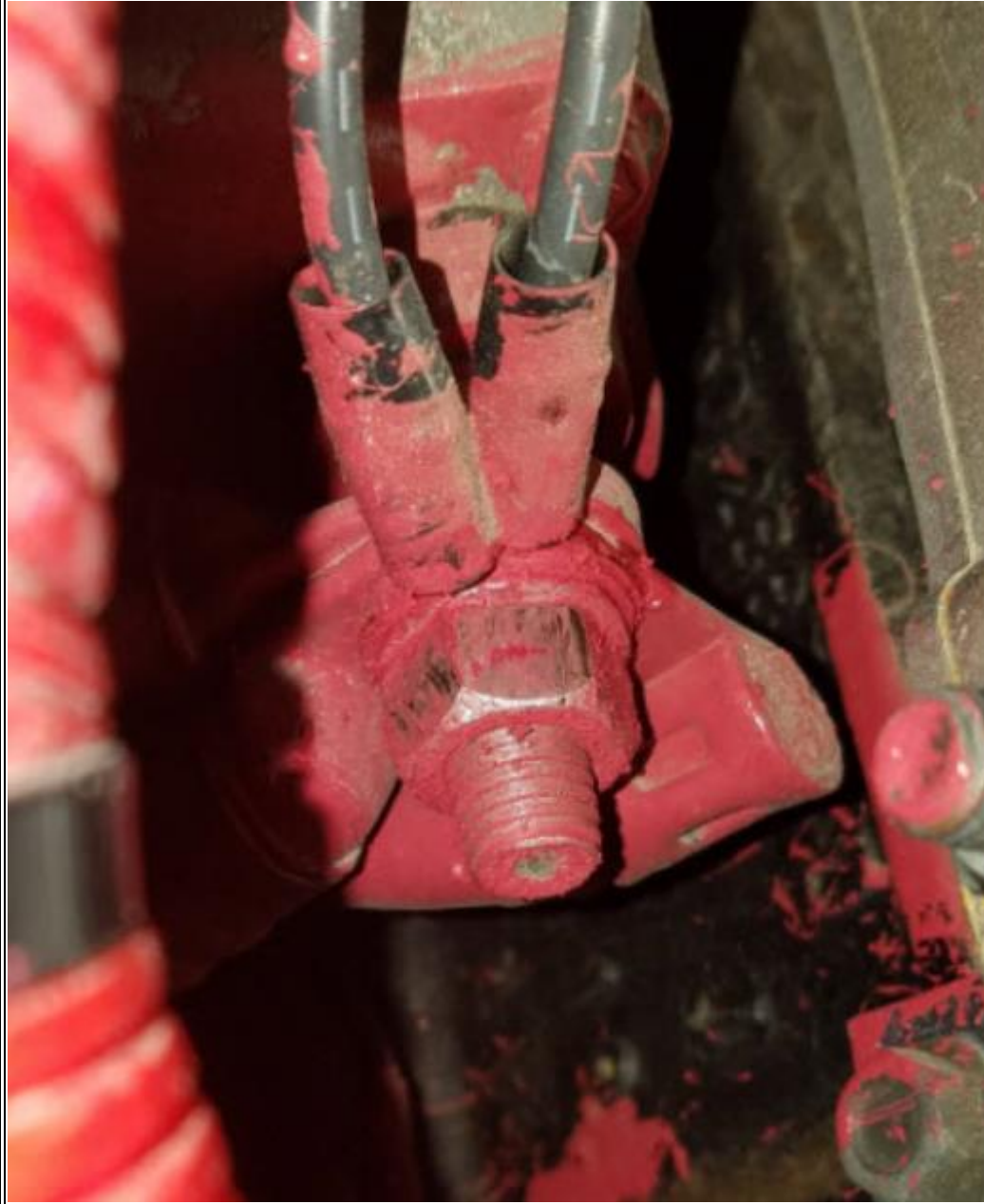
Figure #2: Coating Thinned/Removed via Wire Brush/Scraper
